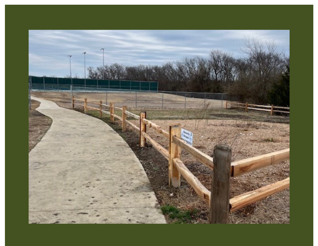
SPLIT RAIL FENCE INSTALL AT THE PARK AT STONE CREEK (PRARIE LAND AREA)
